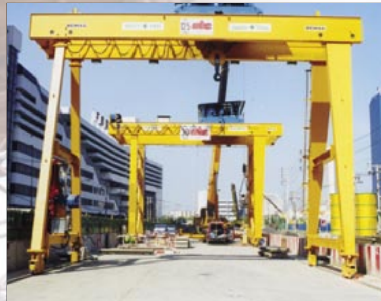
2 units of 70t x 20m double girder full portal cranes used for the construction of a tollway in Bangkok, Thailand.
