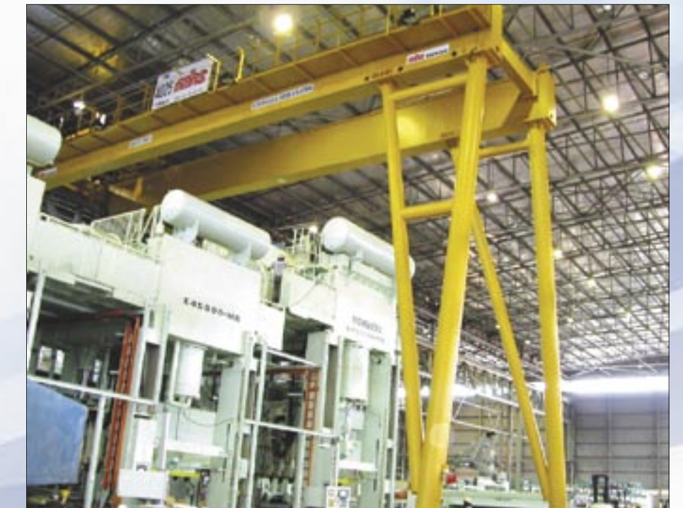
A mould-changing semi-portal crane in an automotive plant.
