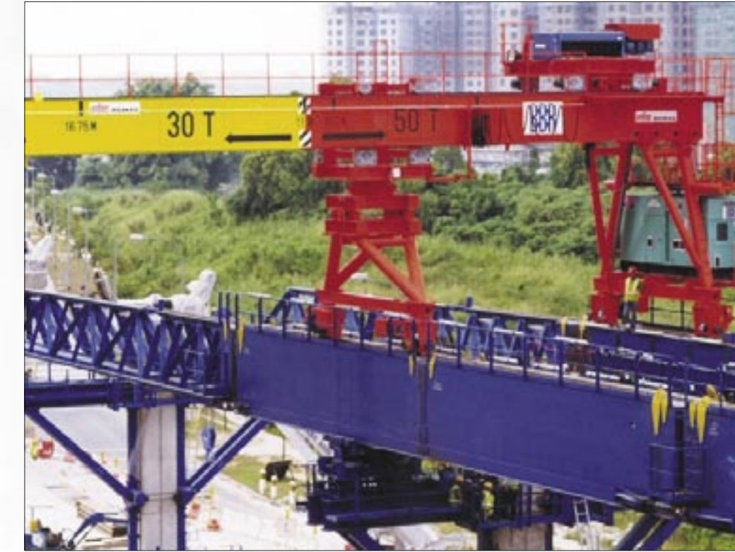
A specially designed crane for the construction of light rail train concrete structures. The crane can negotiate curves with varying span.
